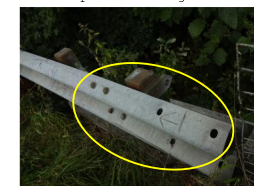
15. View showing missing bolts at parapet/barrier connection
