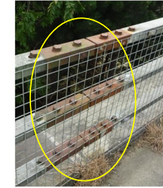
10. View showing typical rusting of bolts and railings
