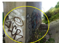
14. View of NE pier showing graffiti
