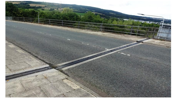
2. View of carriageway looking West showing joint
