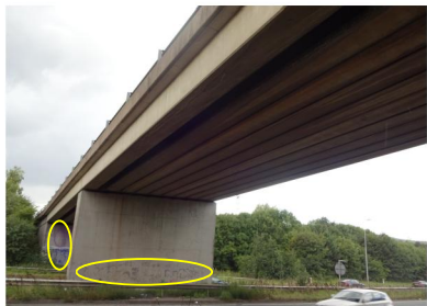
6. General view of soffit showing graffiti on piers and abutment
