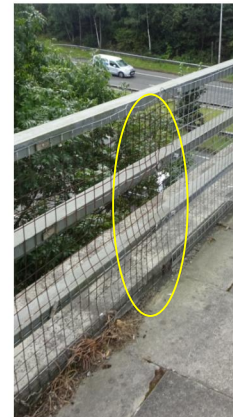
8. View showing damaged mesh along railings
