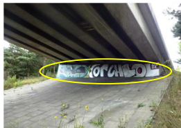
13. View showing graffiti at NE abutment
