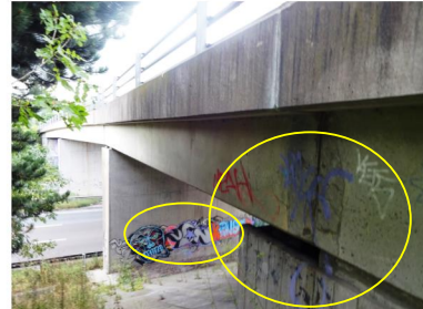
7. General view showing cracks & graffiti
