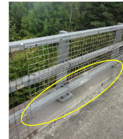
9. View showing missing mesh panel along railing
