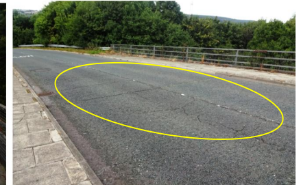
5. View of carriageway showing map cracks
