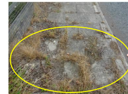
16. Overgrown vegetation on footway
